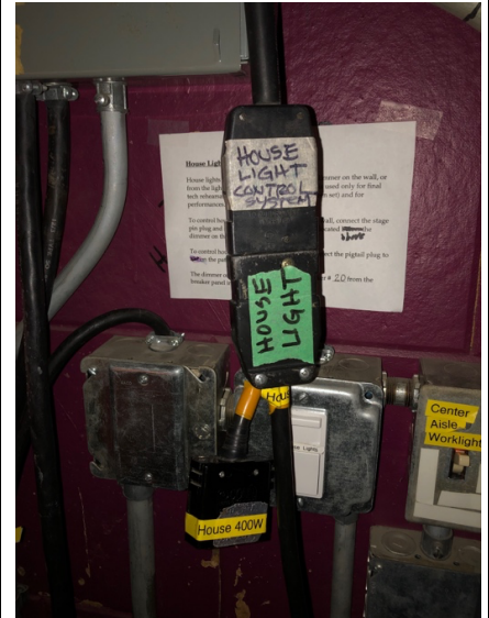
Lighting Control Board Setup
